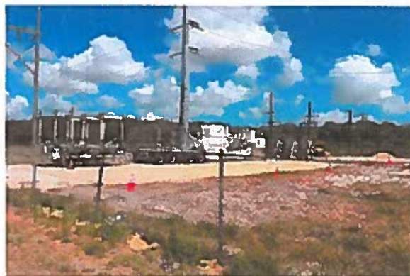
New Portable Substation Installed
