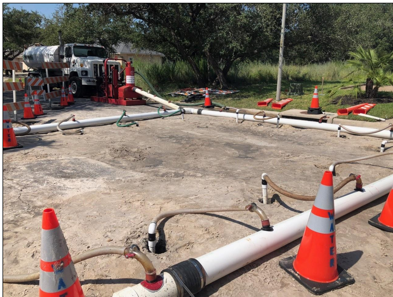
THE SINK HOLE IS TO THE RIGHT OF THE MANHOLE COVER.
